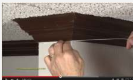
OFS InvisiLight Fiber Installation
